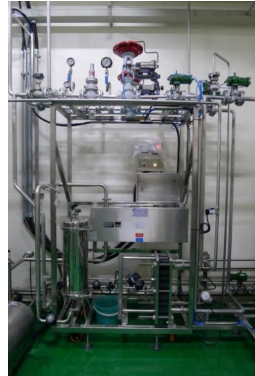
純水循環管路及冰水/熱水站 Pure water circulation system and cool/hot water station
