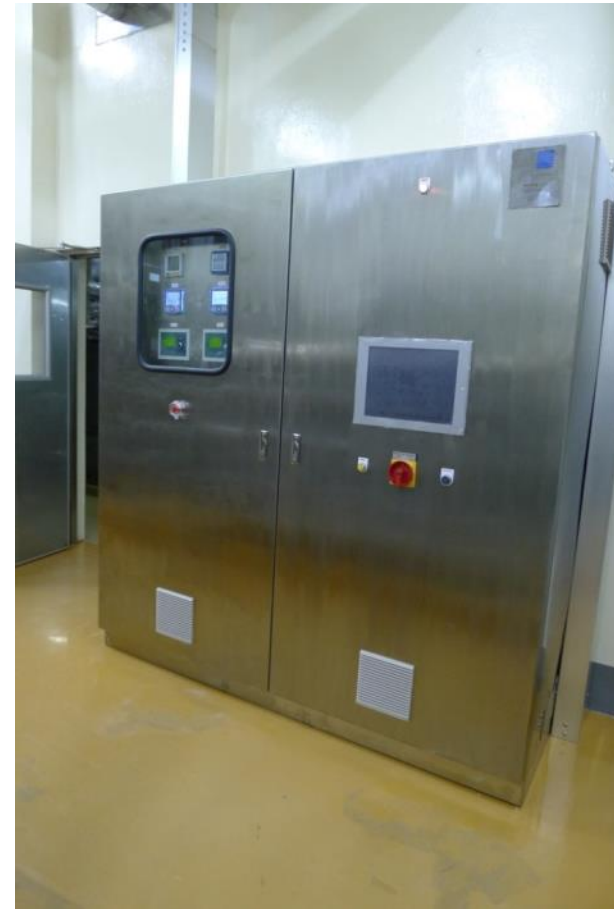
中控盤 Central control panel
