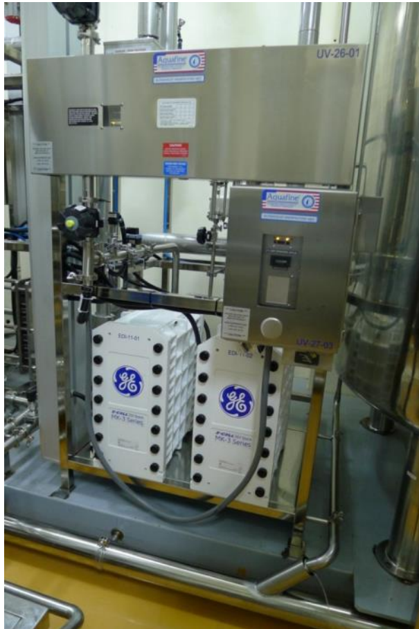
EDI 熱消機組 EDI system (Hot water sanitation)
