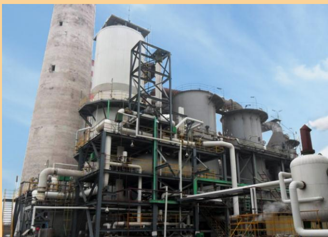
贵州翁福集团公司 2 x40 万吨/年硫磺制酸 HRS 装置技改工程 2*0.4 Million tons /year Sulfuric Acid with HRS Reconstruction project of Guizhou Wenfu Group
