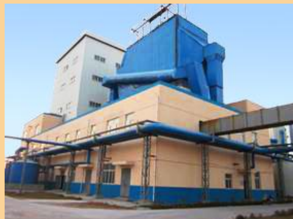
220tds/d Reed Pulp Black Liquid Alkali Recovery Boiler Combustion Workshop Section of Shengda Group Jiangsu Shuangdeng Paper Co.Ltd
